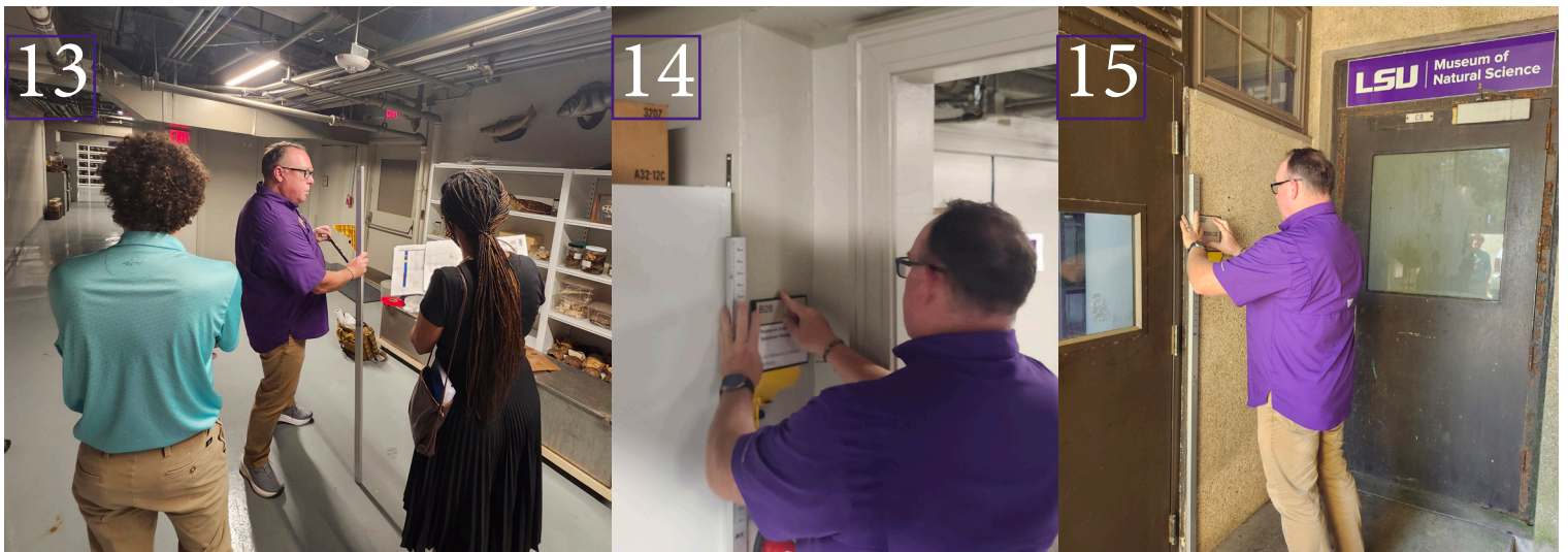
Figs. 13-15: Snapshots capturing the installation of Braille signage in the basement, both indoors and outdoors.
